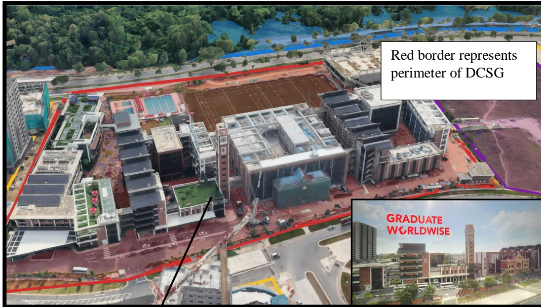
Figure 6 - 3D view of DCSG (Google Earth) during construction, post-construction picture in the bottom right (Dulwich College Singapore)
